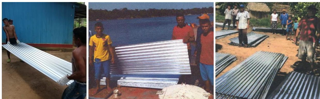
Illustration 83. Sheets of zinc to improve the quality of roofs in homes in RIU-SM
